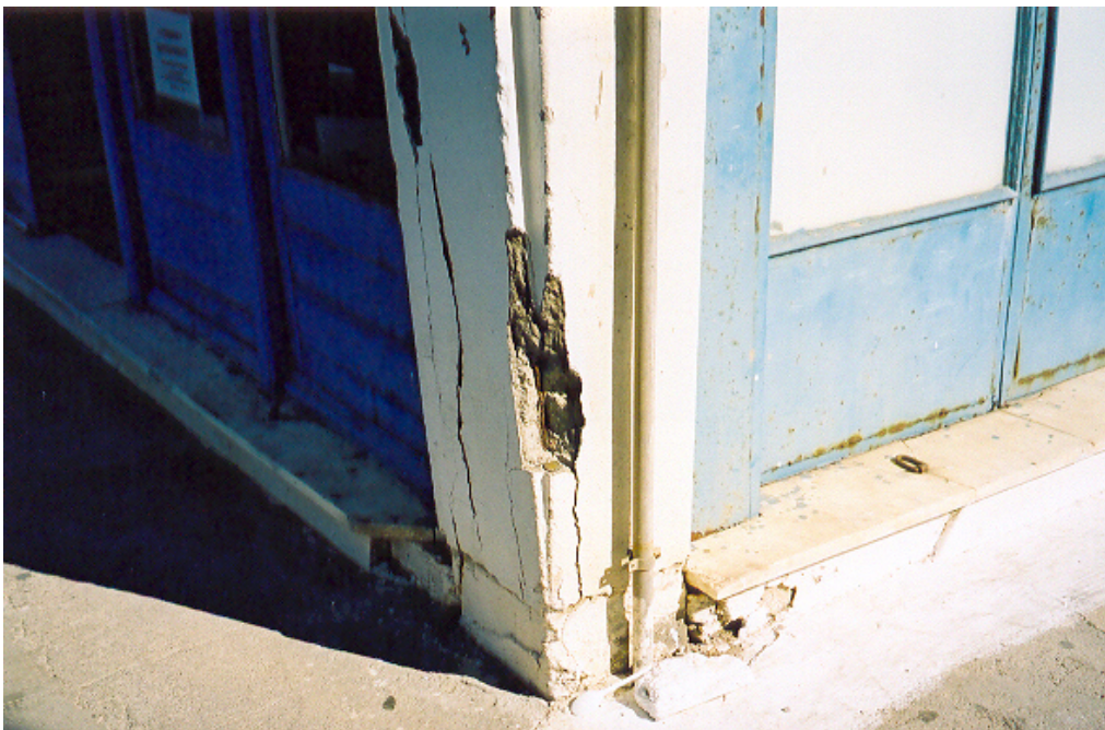
Figure 6.1.1 Photo of deteriorated concrete element due to reinforcement corrosion induced by chloride attack.
